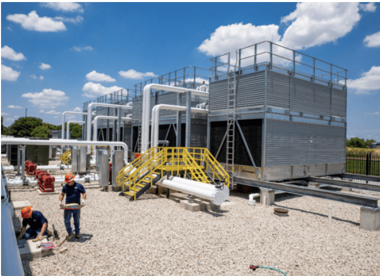
➤ (TOP) Hybrid and Adiabatic Cooling ➤ (BOTTOM) Evaporative Cooling
